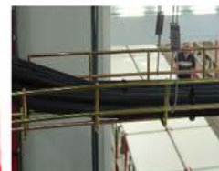
HANGING CABLE TRAY
